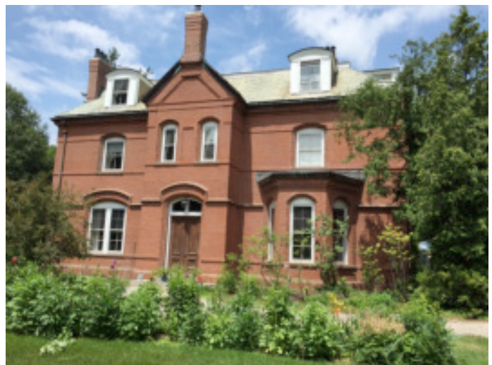
Abbot performed brick restoration on the north (left) side and west (front) sides of the house in separate phases. As evidenced by the photograph, the appearance of the brickwork is identical demonstrating the consistency and quality of the workmanship throughout the both phases.
