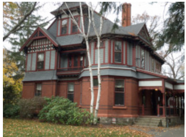
Abbot was contracted to cut and point all of the brick, seal around the perimeter of the windows, and perform masonry work on the foundation.
