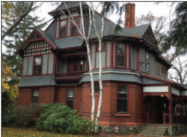
Victorian house in West Newton, Mass.: Abbot was contracted to cut and point all of the brick, seal around the perimeter of the windows, and perform masonry work on the foundation.
