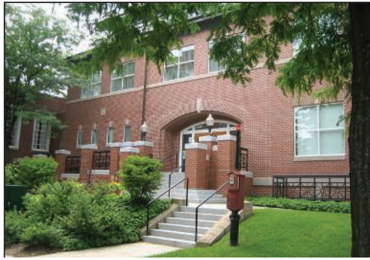
Abbot worked in conjunction with Silverman Trykowski Associates to perform a major restoration of the masonry entrance to the library at Eastern Nazarene College in Quincy, MA.
