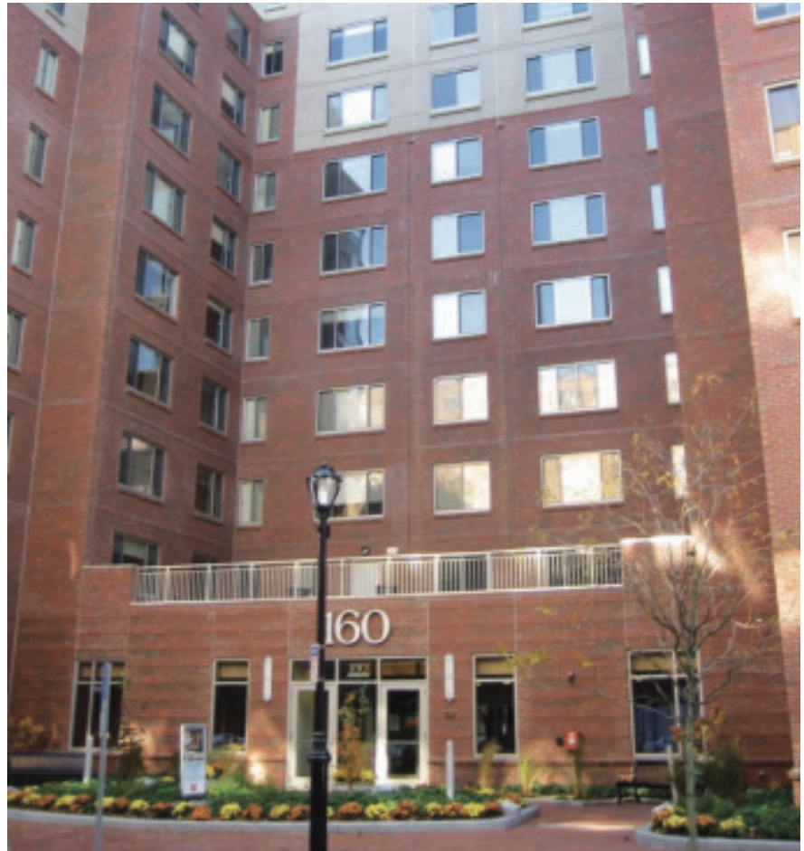
Abbot Building Restoration removed and replaced weatherproofing sealant at the Pleasant Street Apartments in Malden, Mass.
